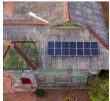
Off Grid Roof Mounted Solar
